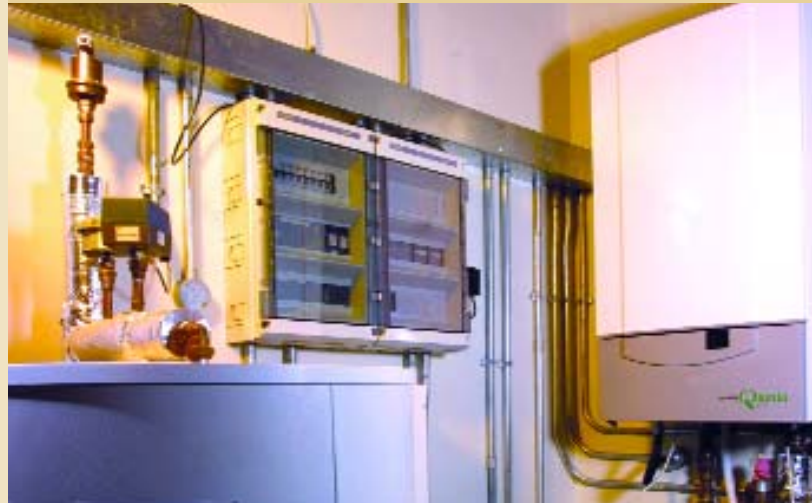
Any type of boiler can be controlled.
