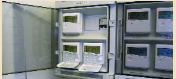
smartZone controllers in a concealed smartBox unit.
