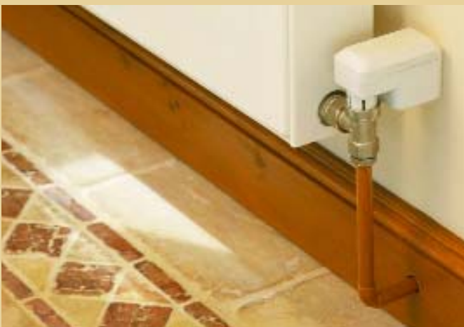
smartcontrols feature project: wet radiator control, country mansion, Hampshire.
