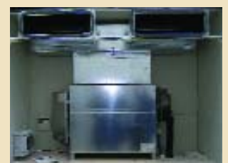
Concealed VRV ducted air-conditioning unit brings comfort cool air into the space.
