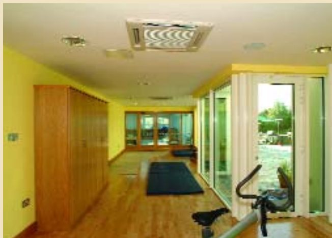
smartcontrols feature project: air-conditioning control, Clanrickarde, Ireland.
