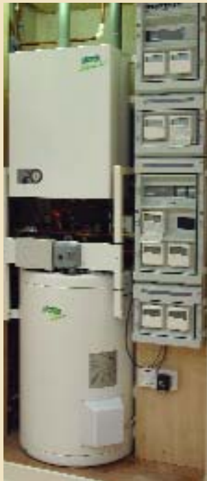
Each piece of equipment is wired to a smartBox control panel.
